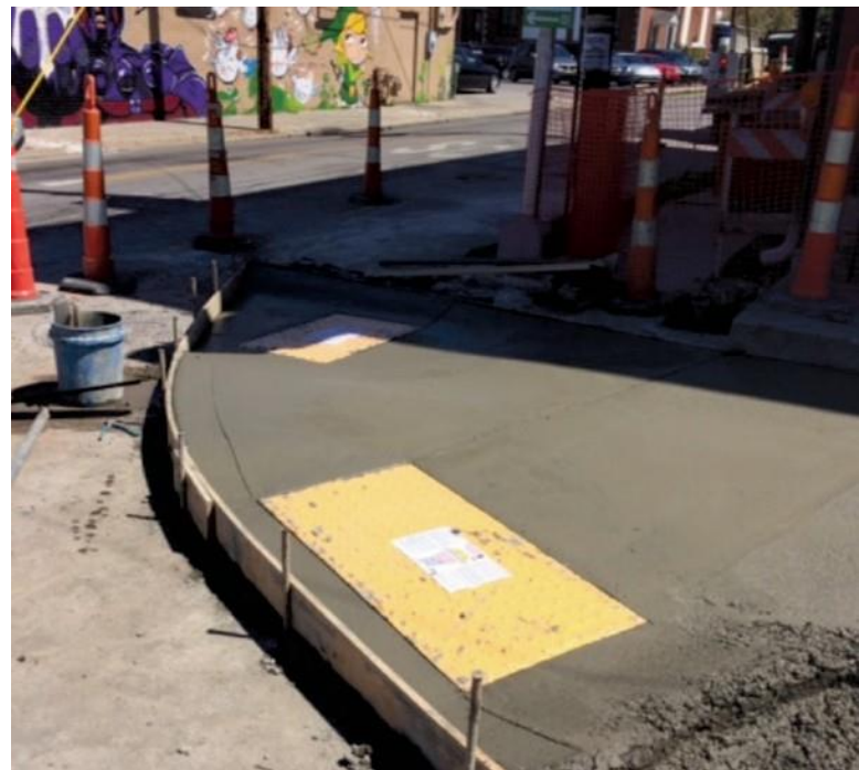
Pedestrian Safety Improvement under construction at 6th Street and North Limestone in Downtown Lexington, KY.
